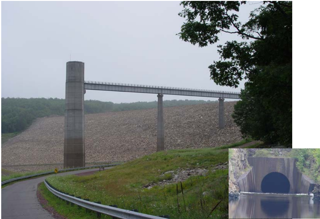
Figure 10-12. Francis E. Walter Dam located in Whitehaven, Pennsylvania. Concrete outfall structure located on the downstream side of the dam is shown at bottom right.
