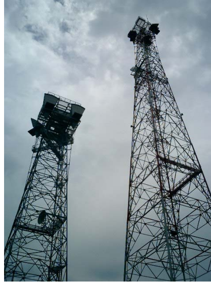
Figure 7-7. Steel tower structures requiring line-line intersections to compute center coordinates based on coordinates observed on each tower leg
